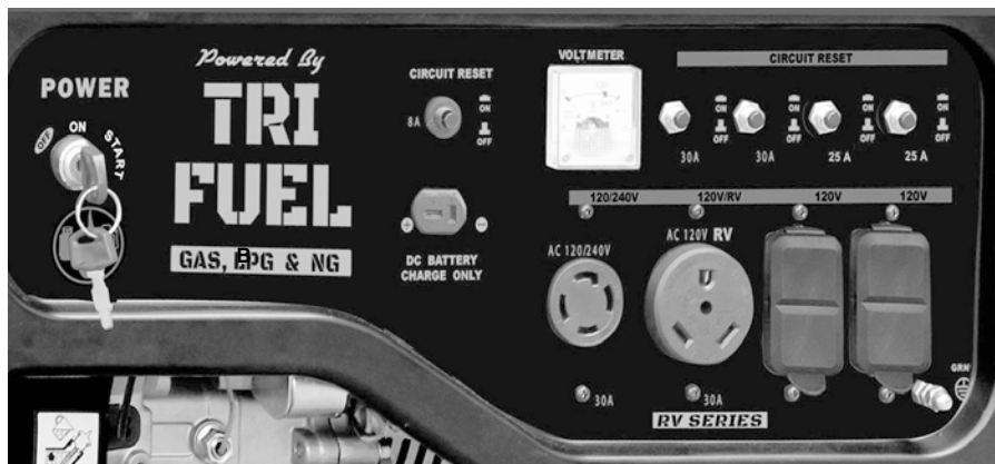
Figure 8 - Outlets available on this generator, from left to right: 12V DC, 120/240V AC, 120V AC RV, and 4 each 120V AC GFCI.
