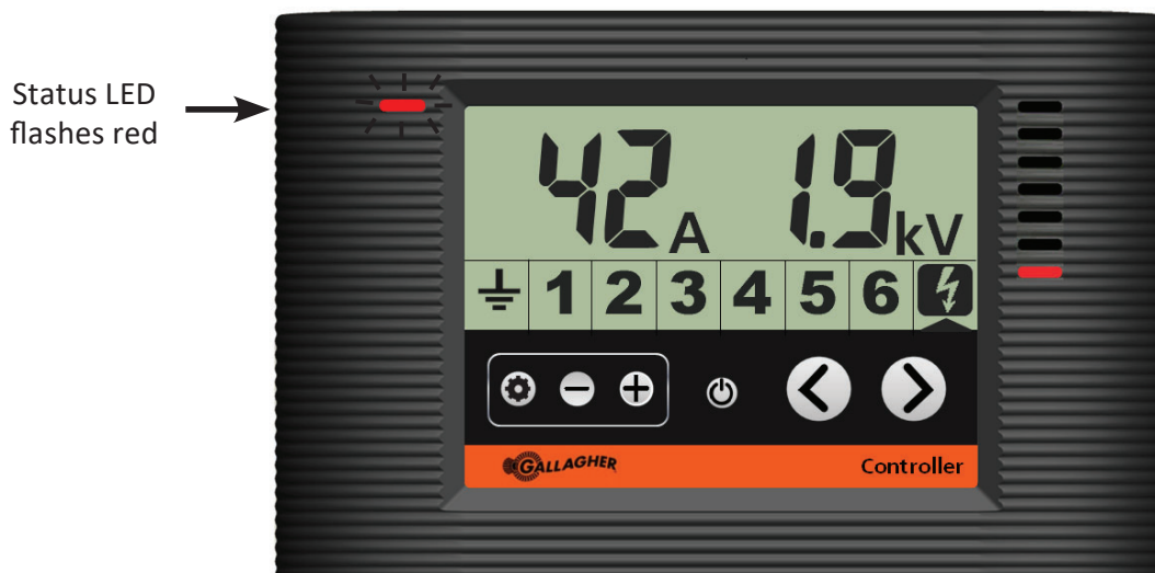
Controller showing the energizer in output alarm
