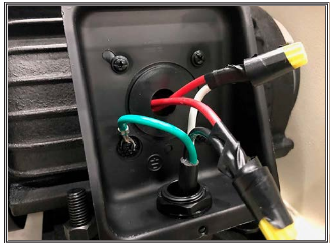
Figure 69. W1865 motor junction box.
