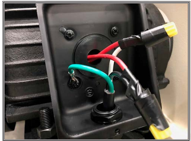
Figure 65. W1864 motor junction box.
