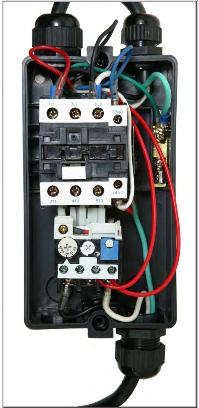
Figure 43. W1754 magnetic switch assembly.
