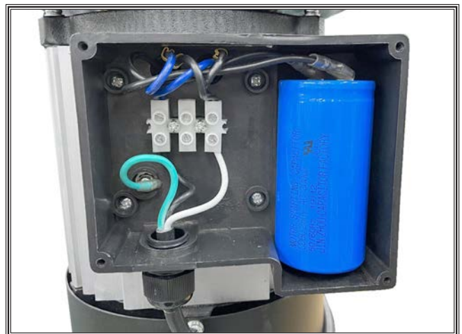
Figure 48. Motor junction box wiring.
