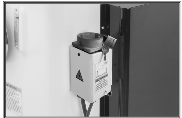
Figure 11. Spindle switch installed.
