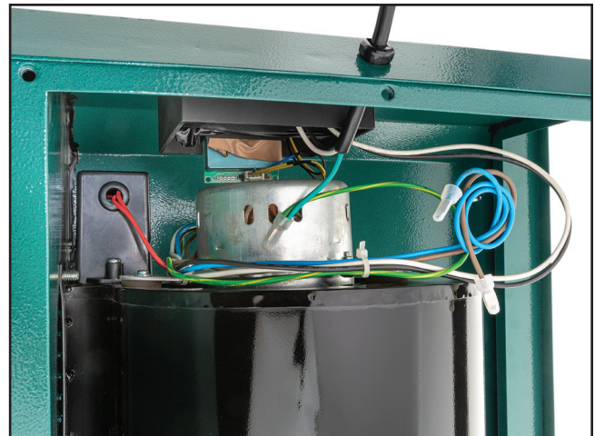
Figure 28. Motor and circuit board wiring.
