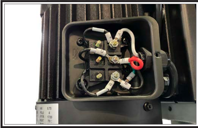
Figure 70. Motor junction box wiring.
