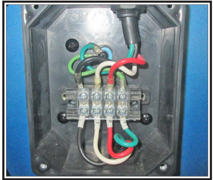
Figure 117. Power supply junction box (220V).
