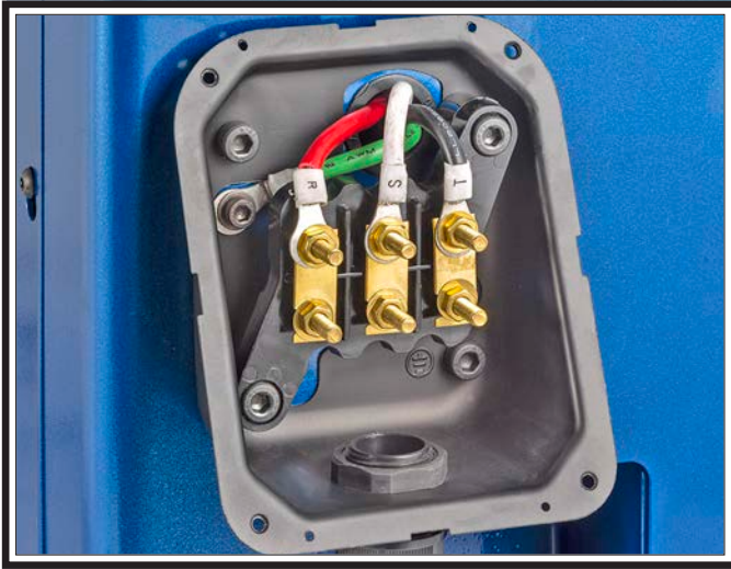
Figure 81. Power supply junction box (220V).
