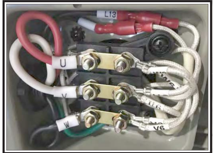
Figure 15. Spindle motor junction box.
