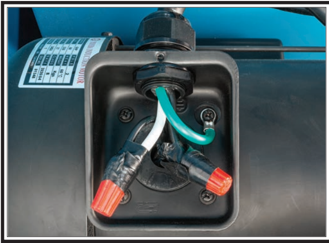
Figure 68. Motor junction box wiring.
