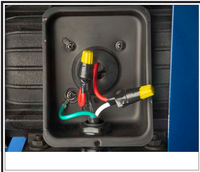
Figure 77. SB1109 motor junction box.
