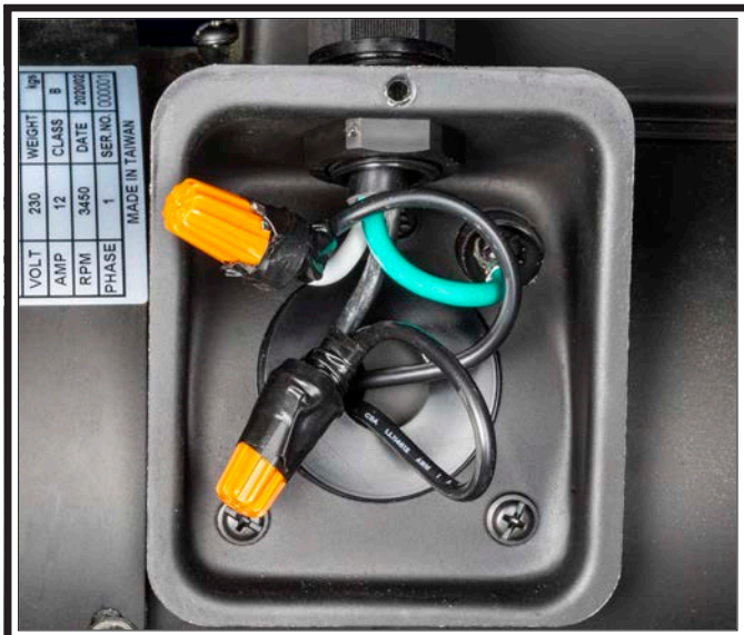
Figure 70. SB1108 motor junction box.
