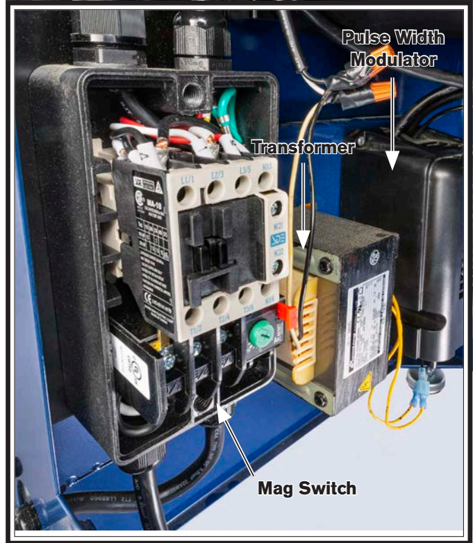
Figure 71. SB1108 mag switch, transformer, & pulse width modulator.
