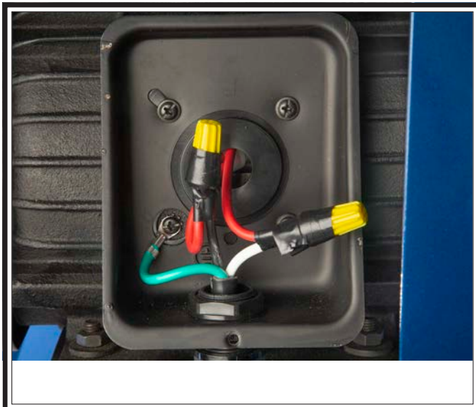
Figure 77. SB1109 motor junction box.
