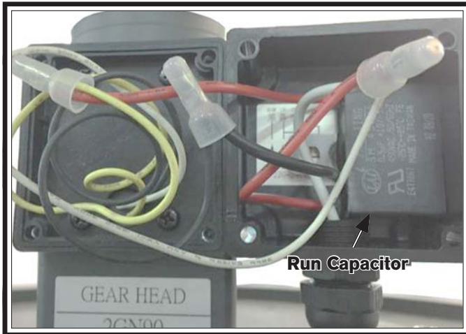
Figure 84. SB1100 filter brush motor junction box.
