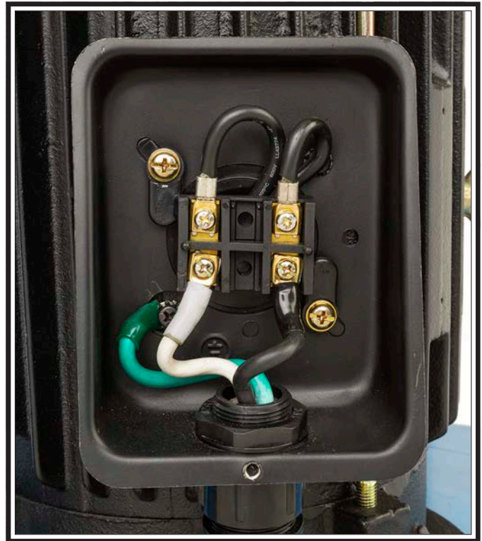
Figure 71. SB1094 main motor junction box.
