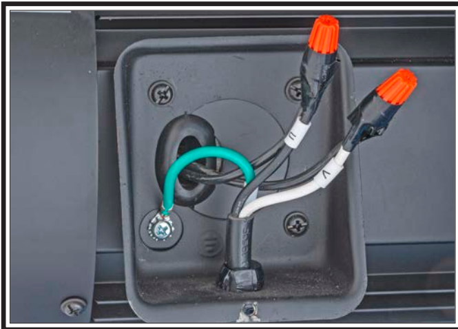
Figure 101. Motor junction box wiring.
