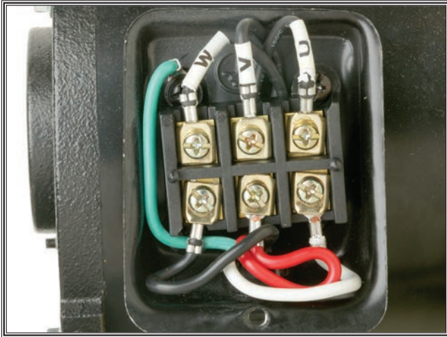
Figure 58. Motor junction box wiring.
