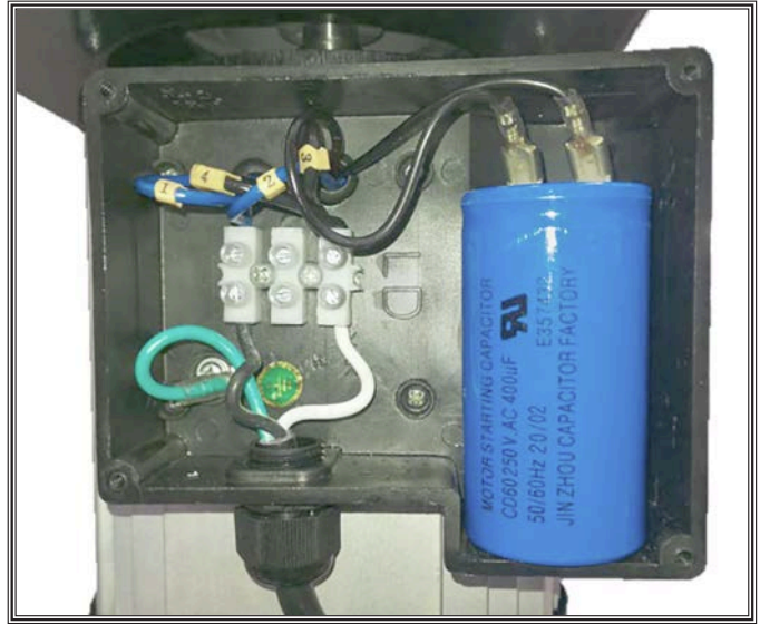
Figure 37. Motor junction box wiring.
