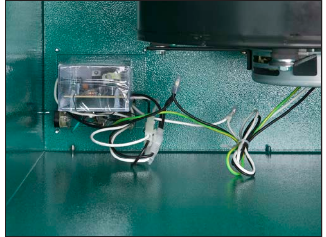
Figure 17. Remote wiring inside view.
