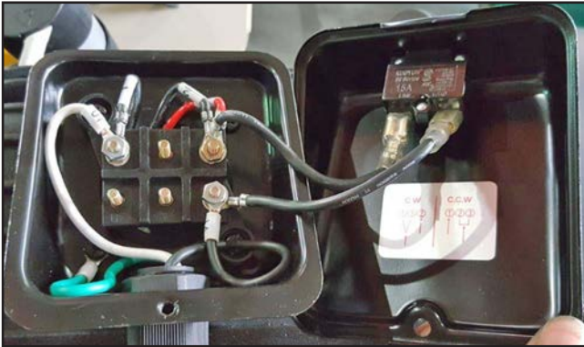
Figure 48. Junction box (M1).
