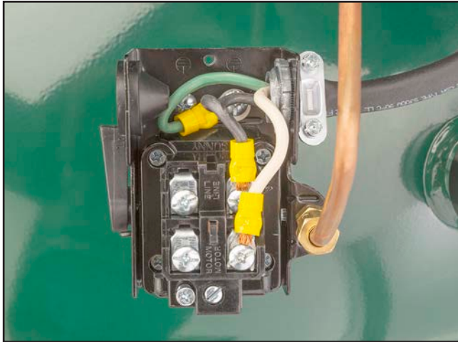
Figure 62. Pressure switch wiring.
