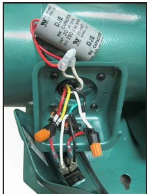
Figure 24. 120V junction box.
