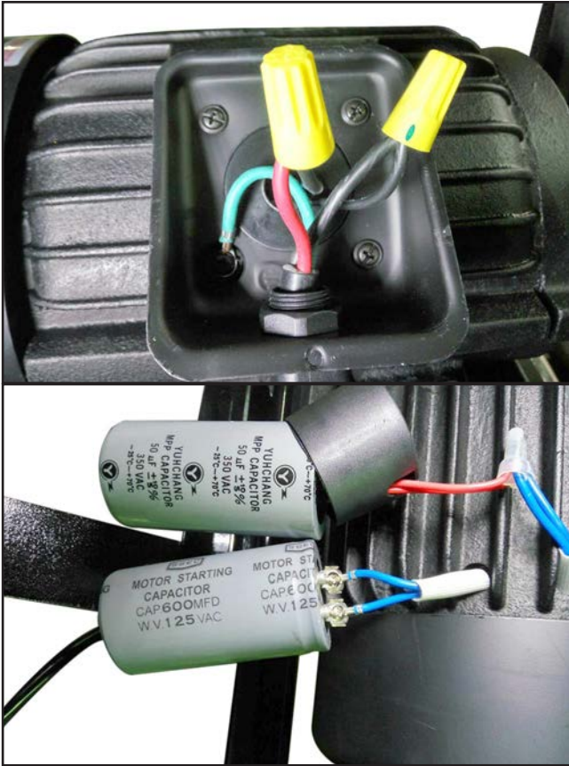
Figure 57. G1066Z drum motor connections and capacitors.
