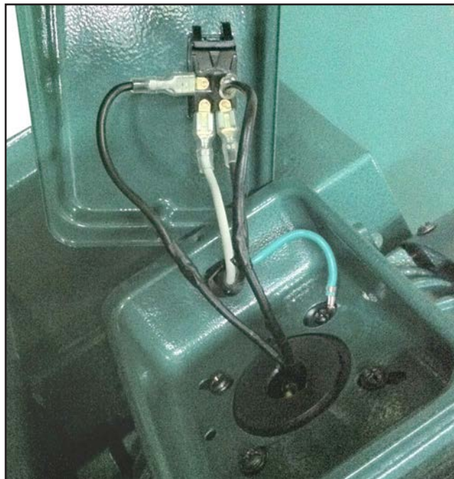
Figure 75. G1029Z2 junction box and switch.
