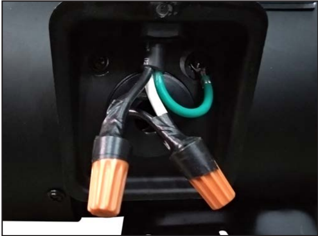
Figure 73. G1021Z motor junction box.
