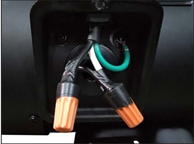
Figure 73. G1021Z motor junction box.
