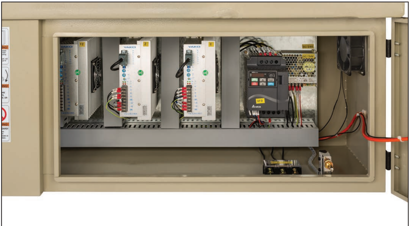
Figure 86. Electrical cabinet components (right).
