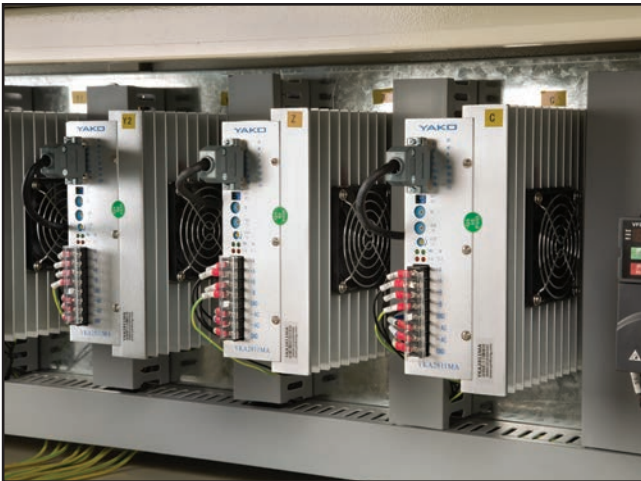
Figure 88. Right electrical cabinet stepper drivers.
