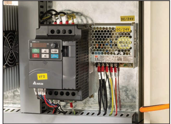
Figure 90. VFD and 24VDC power supply.
