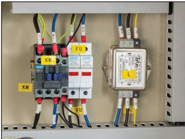
Figure 52. Contactor, fuse holders, and EMI filter.
