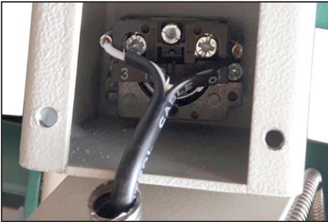
Figure 83. E-stop switch box.
