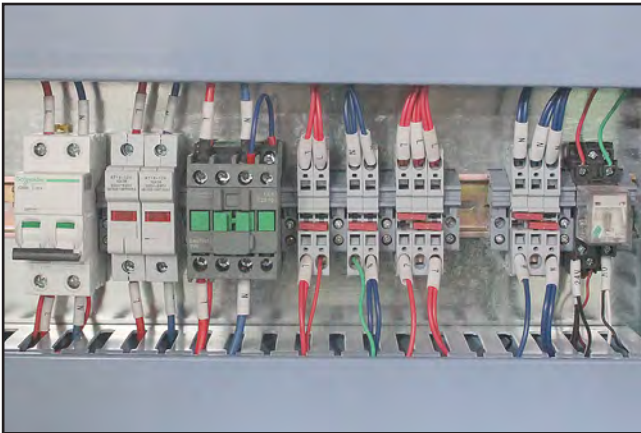
Figure 67. Circuit breakers, contactor, and fuses.
