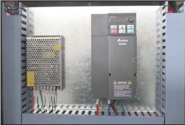
Figure 66. VFD and power supply.
