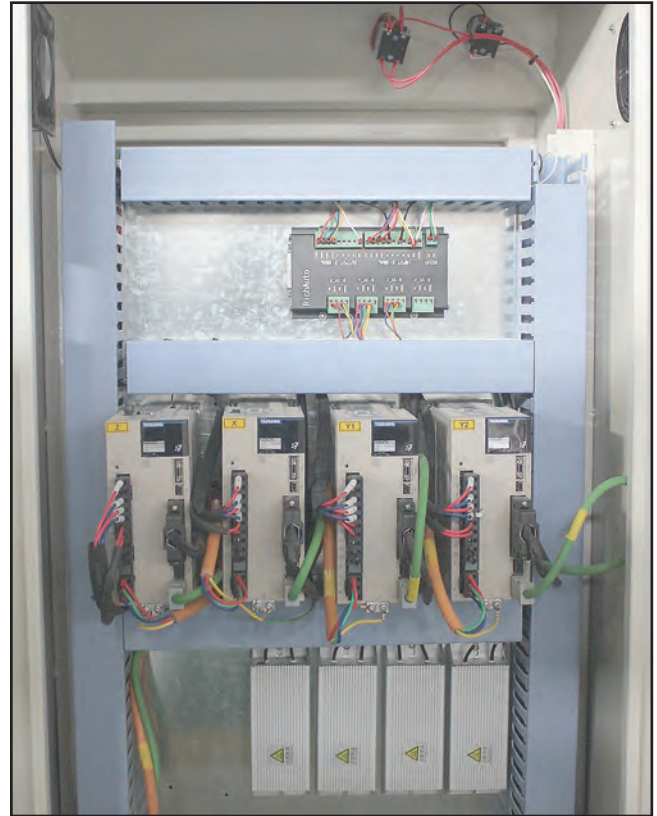
Figure 65. Rear view of electrical cabinet.
