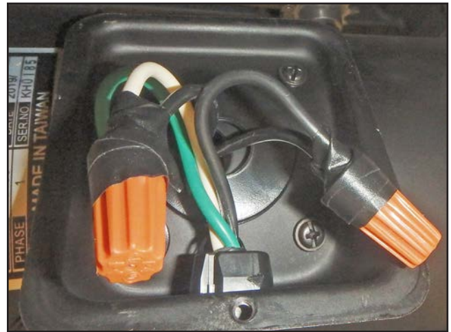
Figure 54. G0890/G0891 motor junction box.
