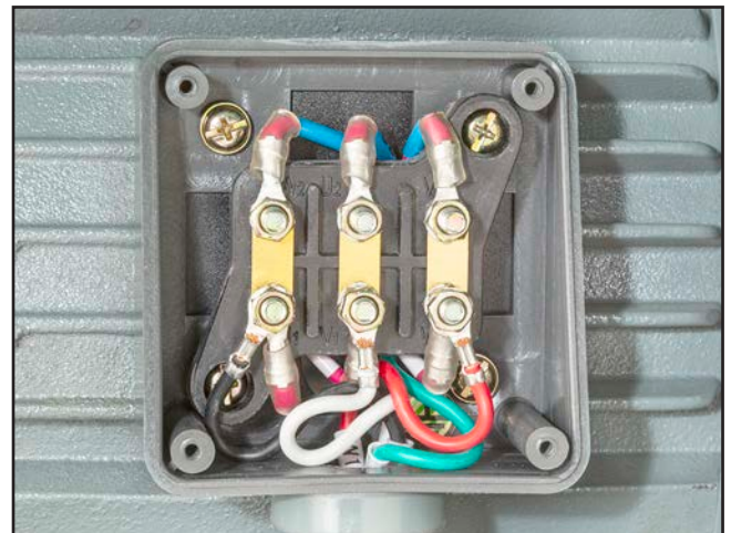
Figure 129. Hydraulic unit motor junction box.
