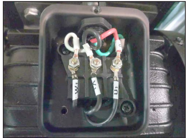
Figure 93. Main motor wiring connections.
