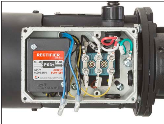
Figure 91. Feed system motor wiring connections.
