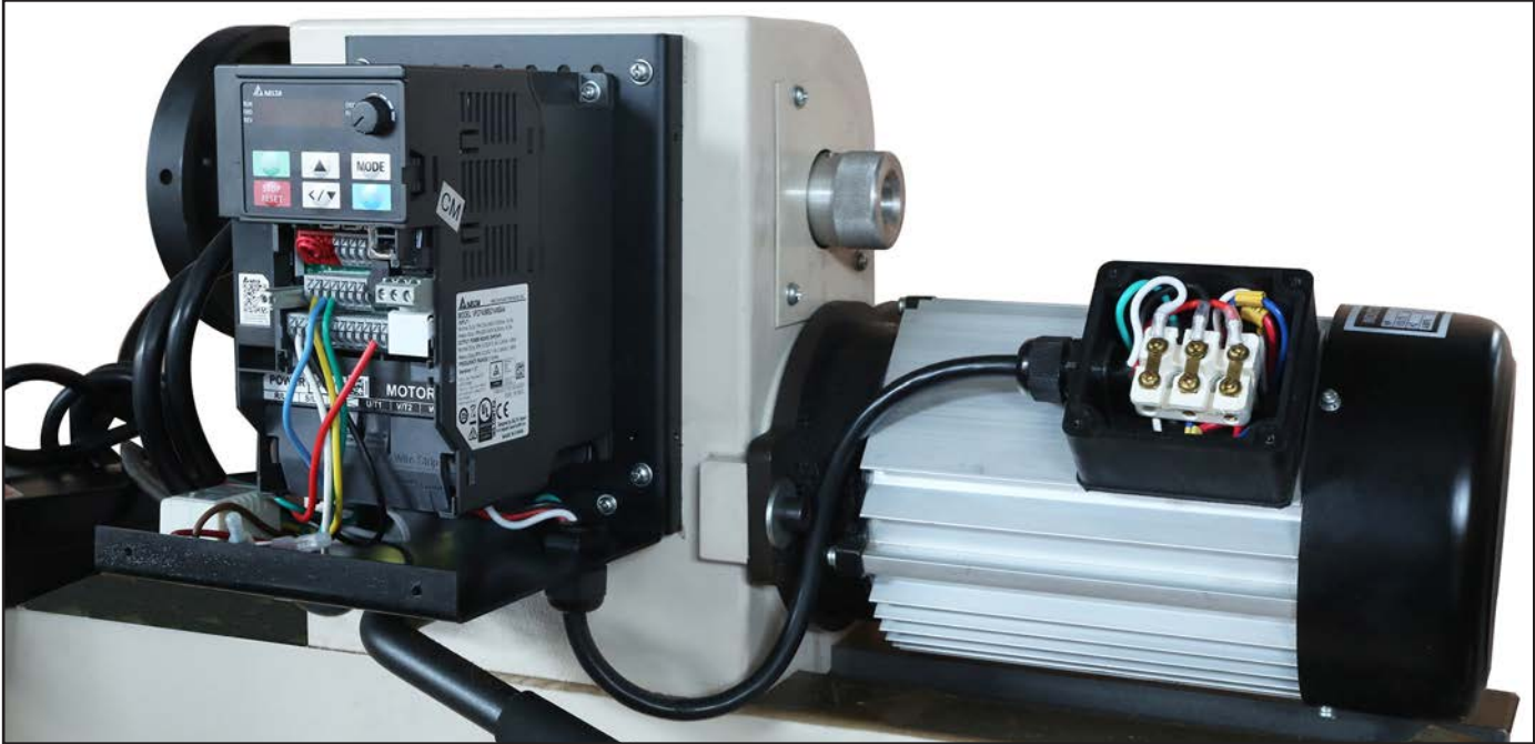
Figure 53. Inverter box and motor junction box locations.
