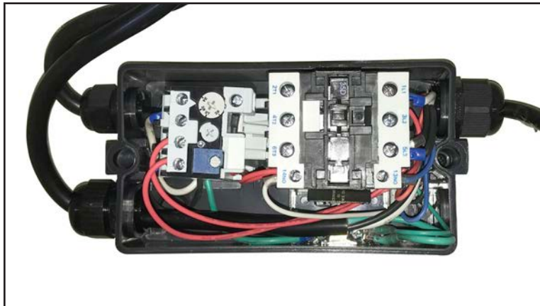
Figure 67. Magnetic Switch (behind control panel).
