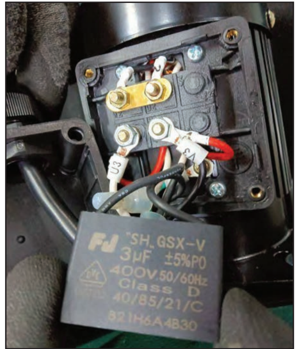
Figure 104. Coolant pump wiring.
