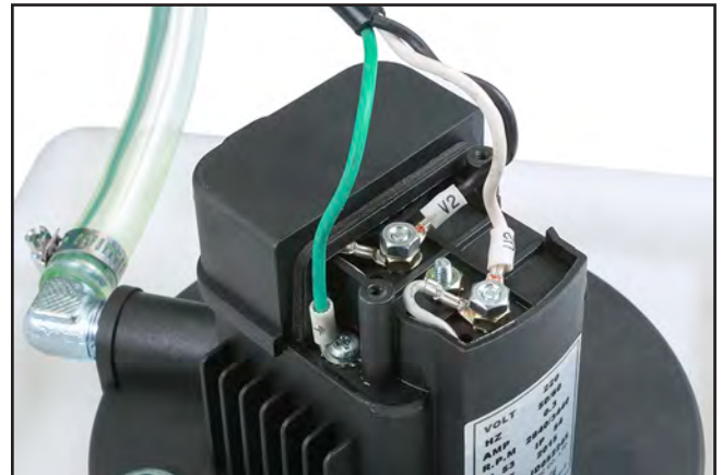
Figure 69. Coolant pump wiring.
