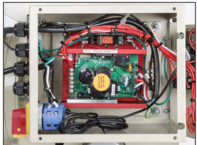
Figure 87. Electrical box wiring.
