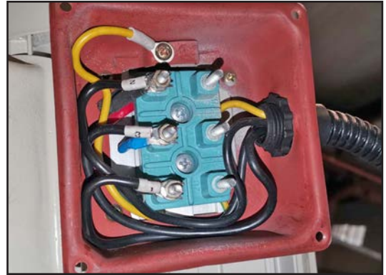
Figure 108. G0796 motor wiring.
