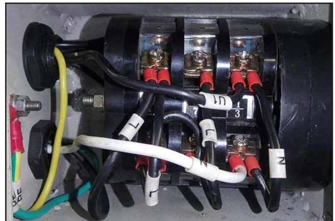
Figure 39. Switch box wiring (left side).
