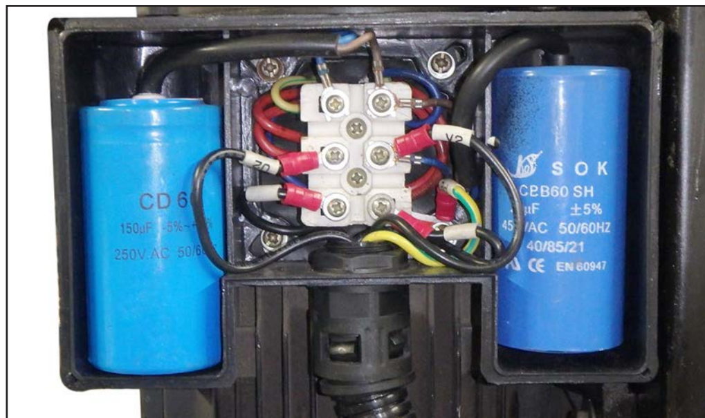
Figure 40. Motor junction box wiring.
