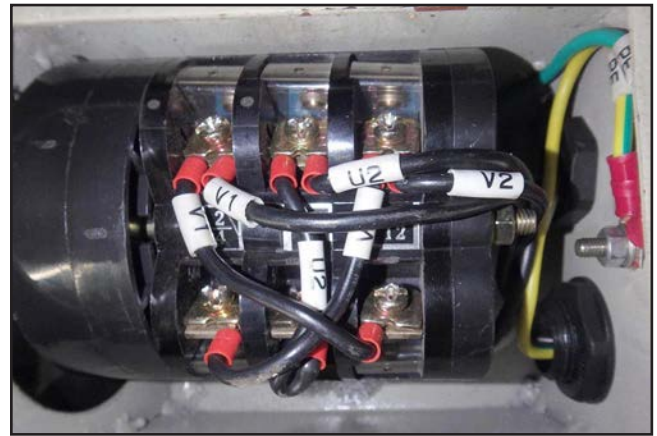
Figure 38. Switch box wiring (right side).
