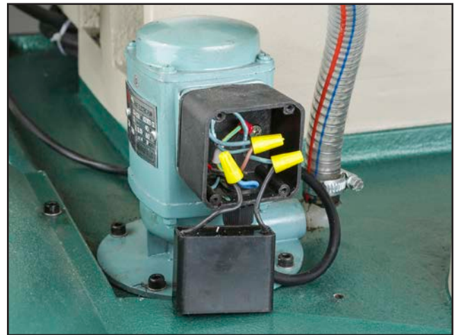
Figure 87. Coolant pump wiring.
