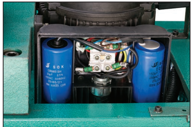
Figure 86. Horizontal spindle motor wiring.
