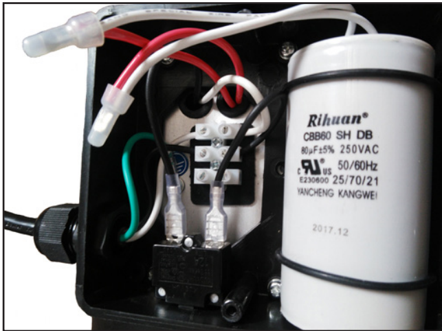
Figure 41. Sanding motor wiring.
