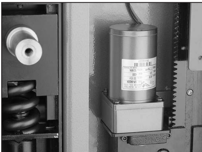
Figure 90. Guide post elevation motor wiring.
