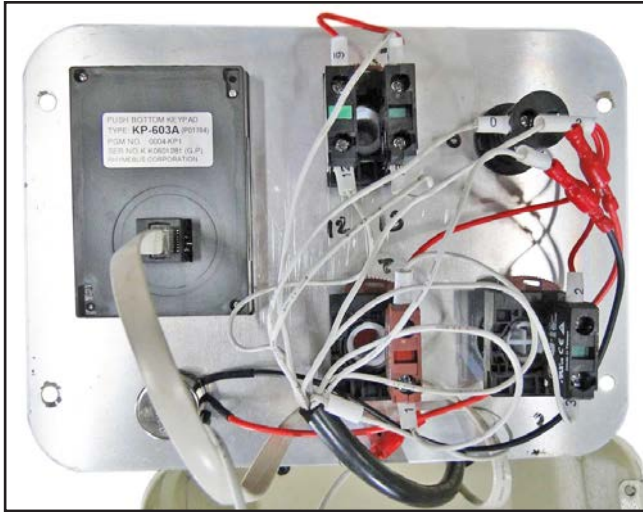
Figure 55. Control panel wiring.
