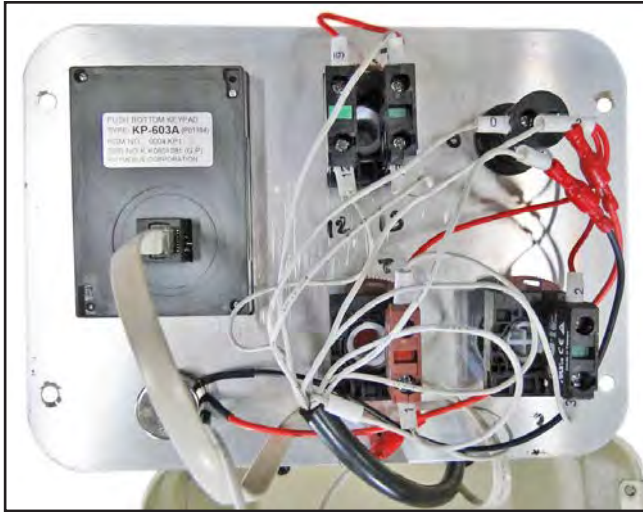
Figure 46. Control panel wiring.
