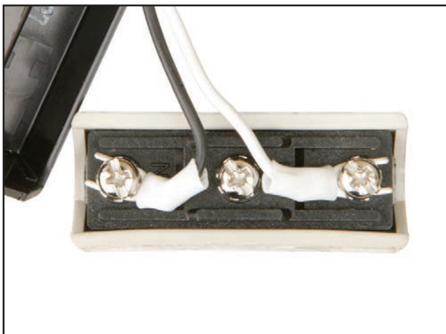
Figure 91. Lower right door safety switch wiring.
