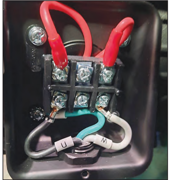
Figure 75. Motor junction box wiring.
