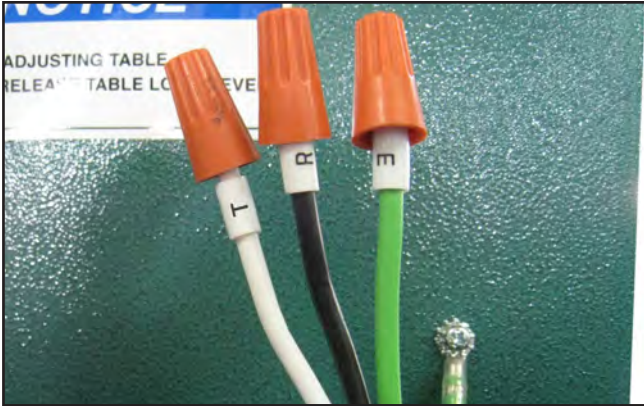
Figure 72. Power supply wiring.
