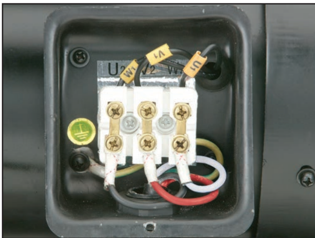
Figure 5. Motor junction box wiring.
