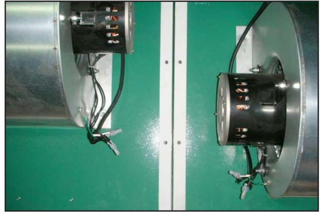
Figure 27. Wiring for both motors.
